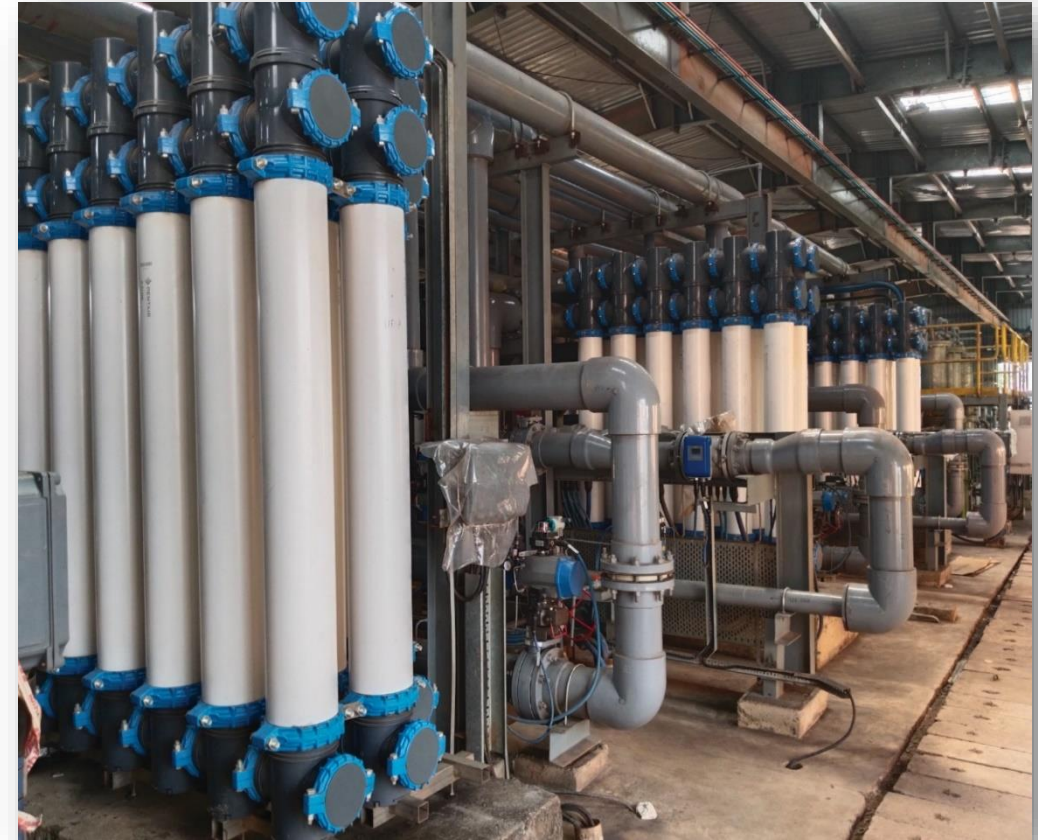
NMDC ZLD Plant, Chhattisgarh, India
