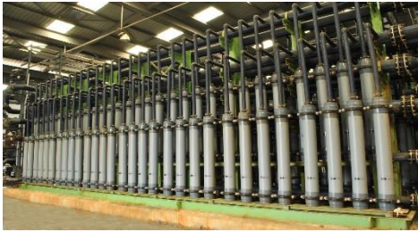
110 MLD SWRO (Desalination) Plant, Nemmeli, Chennai, India India's largest operational desalination plant till date
