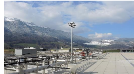
14 Sarneraatal WWTP, Alpnach, Switzerland First plant in Switzerland to be commissioned with NEREDA® technology
