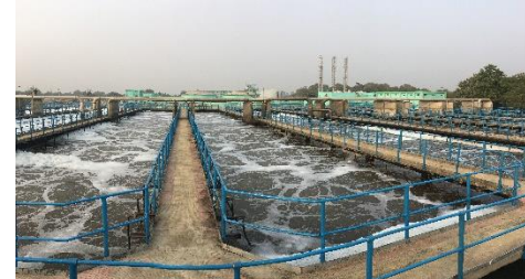
140 MLD Sewage Treatment Plant, Dinapur, Varanasi, India First and largest STP to be inaugurated under 'Clean Ganga' mission
