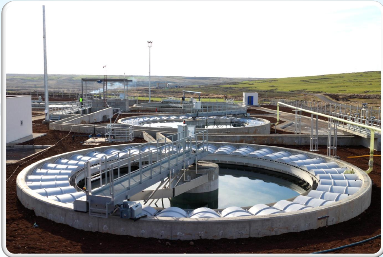
Waste Water Treatment Plant, Siverek, Turkey
