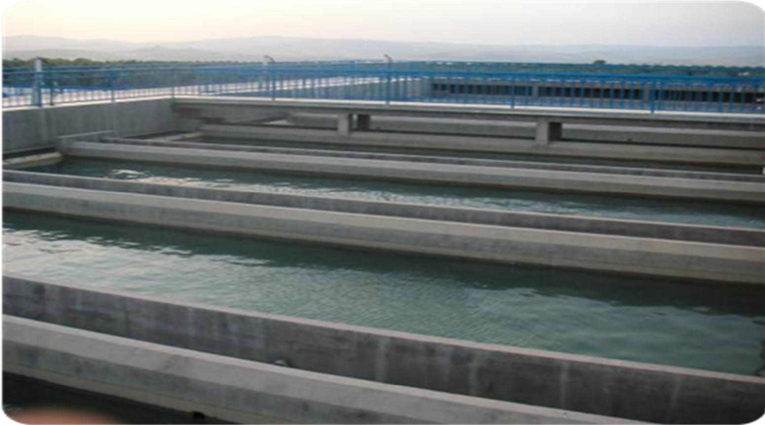
Sidi Abdelli, Algeria Reservoir water treatment, multi-barrier, 95,000 m 3 /d
