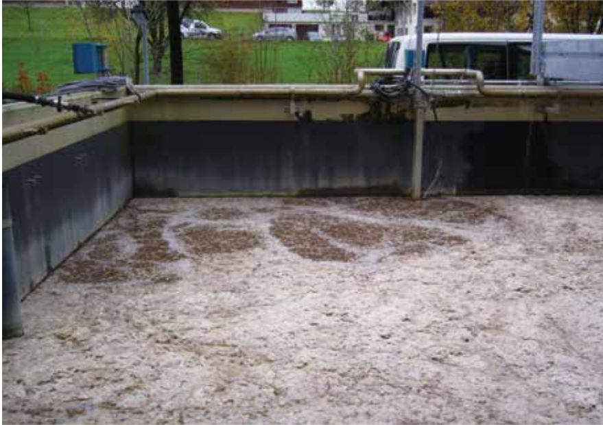
📍 Niederglatt, WWTP, Switzerland
